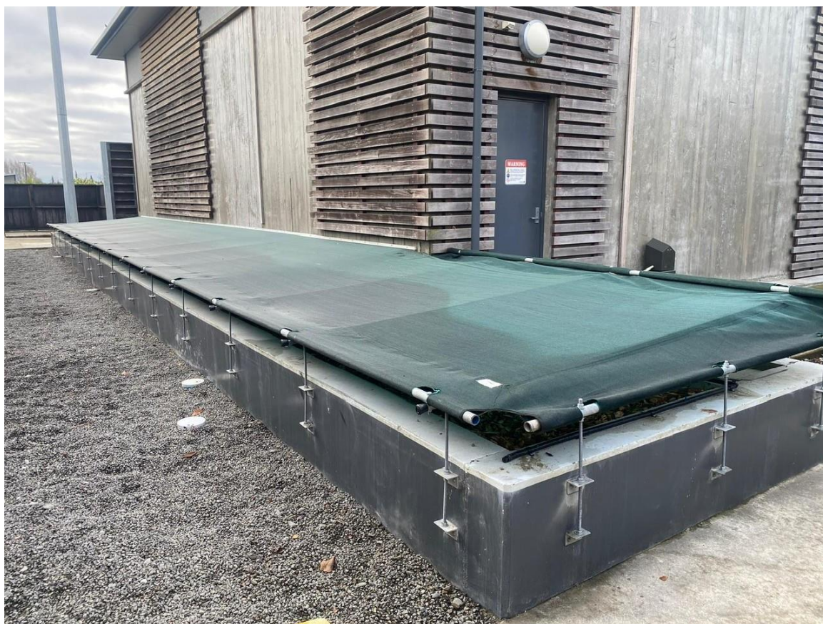
Photo: An example Vacuum Station Biofilter cover at the Prestons Rd Station VS5001.
