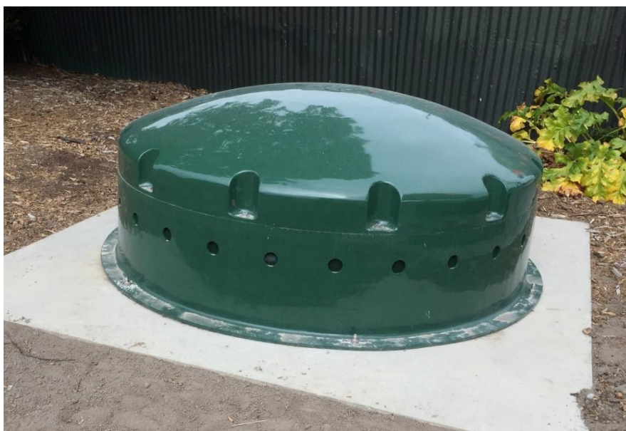
Photo: Western Interceptor Olliviers Reserve Activated Carbon Filter with internal fan and heater. Includes a square concrete base pad extending 200mm beyond the flange base.
