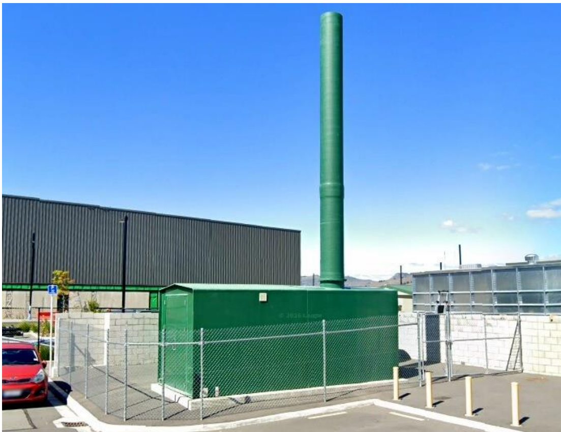
Photo: Balfour Tce Bio-scrubber with Air Dispersion Vent Stack – Station ID: OC0508
