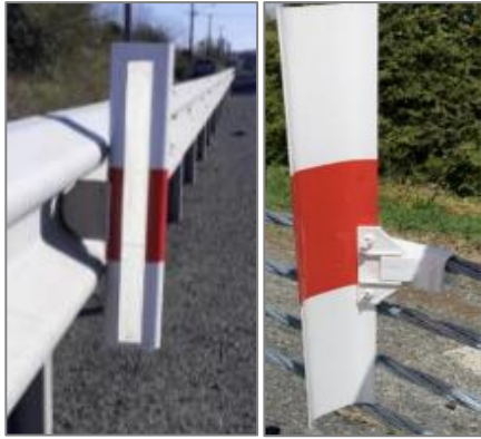
Figure 6: Delineator attached to barrier
