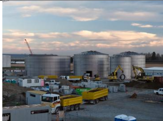
Tank farm installation
