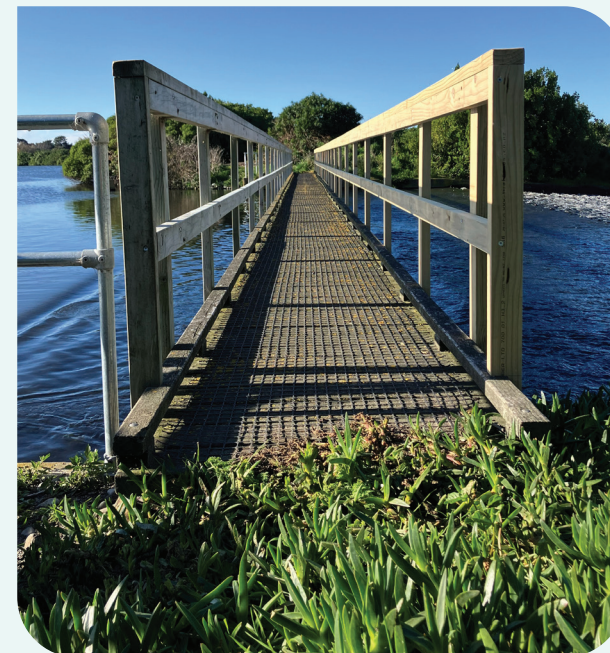
Check out our latest Health and Safety improvements – a new hand-rail on a walkway at ponds and ...
