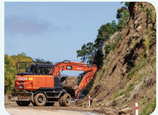
Little River - post flooding.
